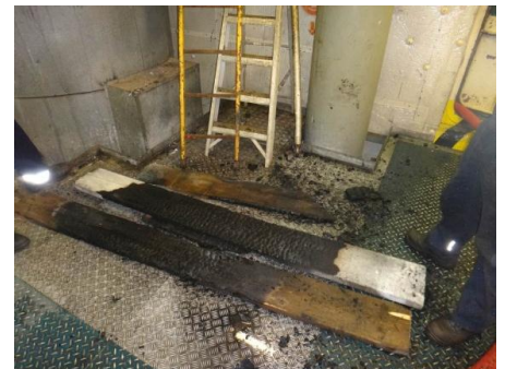
Smouldering scaffold boards
