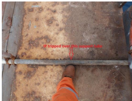
Tripping over scaffold board
