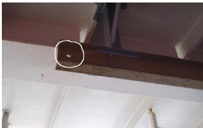
Figure 2 - H-beam with missing 'Trolley Stopper'
